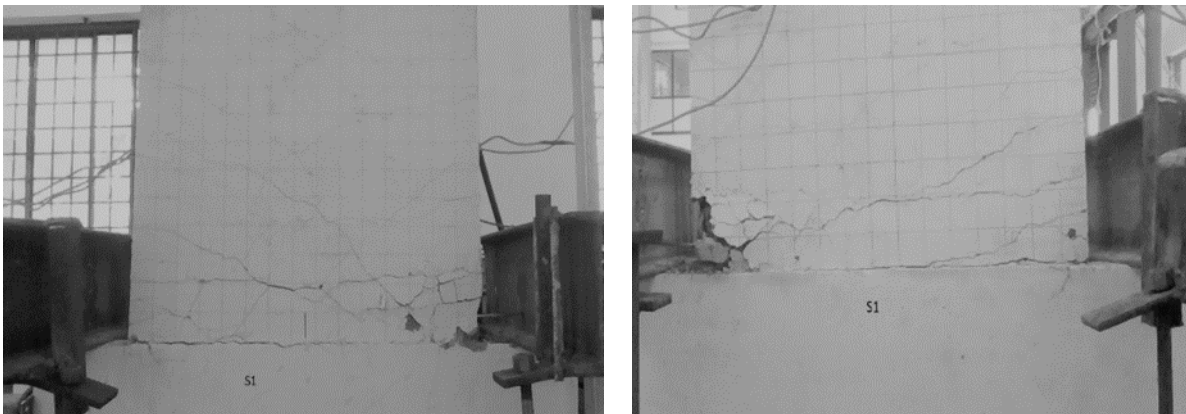
Figure 10 Crack pattern of conventional reinforcement specimen (S1)
