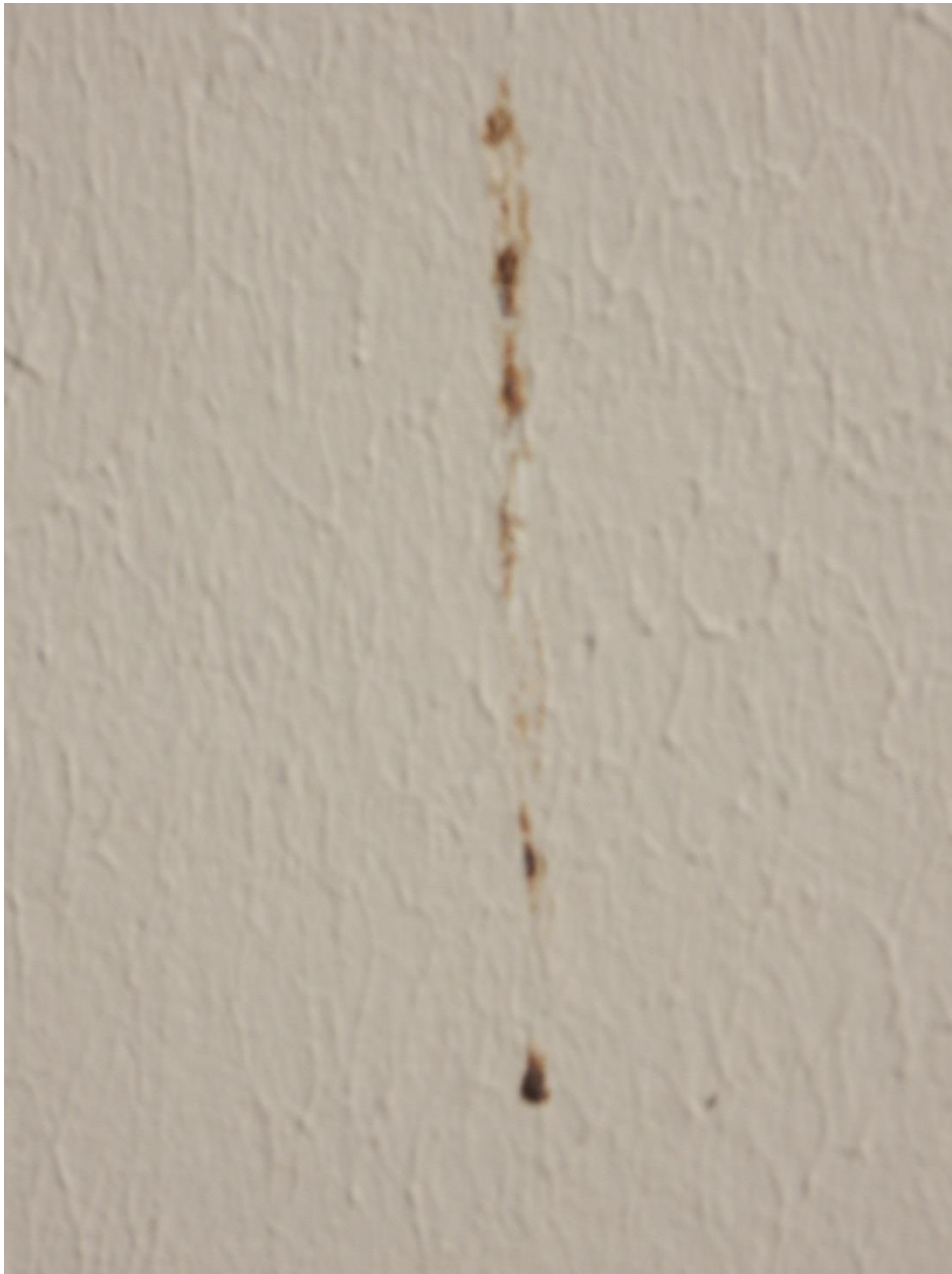
Figure 6 Recent concrete construction showing zero cover to the rebar and the painted surface not preventing the start of corrosion
