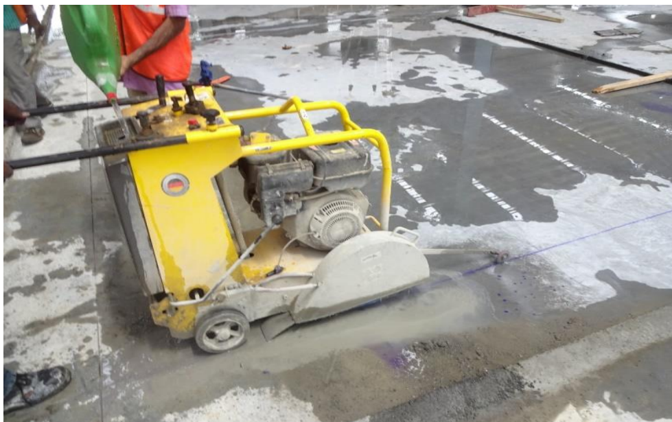
Figure 7 Saw Cutting in Progress, Generally depth of 1/3 of Slab thickness and 35 mm width is cut within 12 hrs
