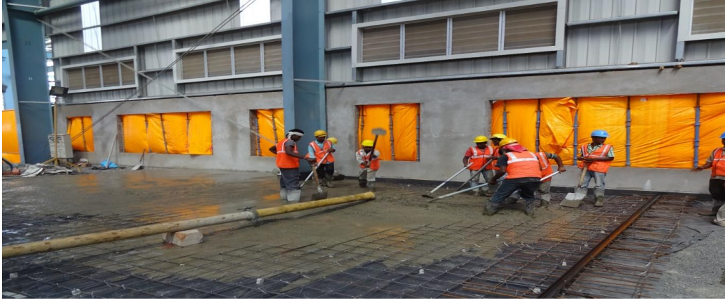
Figure 2 Show the concreting in progress with reinforcement laid and all opening closed for control concrete.
