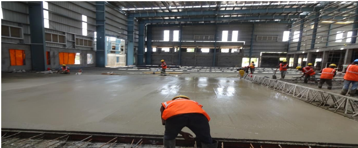
Figure 4 Truss base screed vibrator is run on the Channel both side for proper level and compaction. With Panel Size of 55m (L) X 11.3 m (W).
