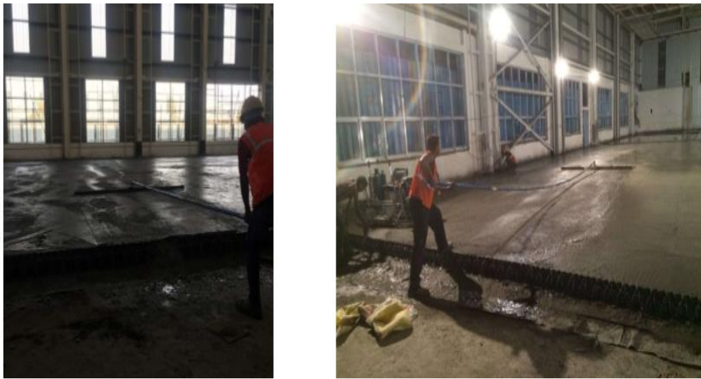
Figure 5 Bull Floater Work in Progress to remove local bumpiness and straightening of the fresh concrete
