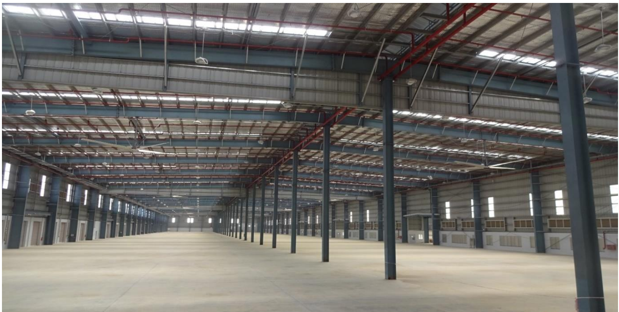
Figure 9 Shows the floor with FM2 Floor with 6.5 mm level tolerance and 2mm flatness tolerance across the floor from Datum
