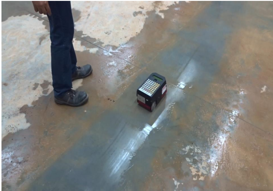
Figure 8 The Profile o graph taking the reading of the floor to check level and flatness. Face Digital Profilegraph within a narrow aisle
