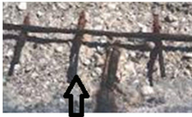
Deterioration due to corrosion
