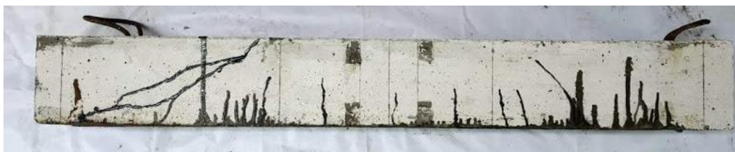
(c) CFRP – 90% DISTRESS
